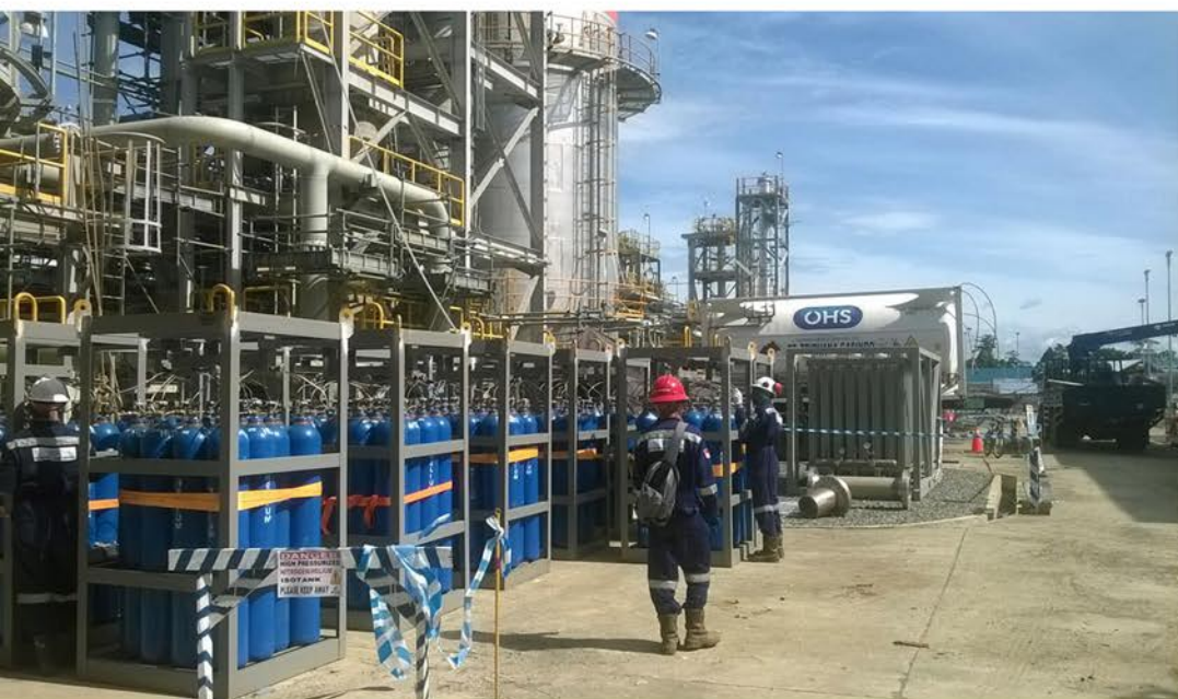
Matindok Gas Development Project
